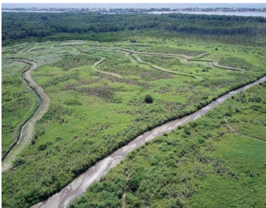
The ecological mangrove restoration of the Puntarenas Estuary in Costa Rica is the largest coastal engineering initiative in Central America. To restore hydrological connectivity, nearly 5 kilometers (3 miles) of channels have been excavated or rehabilitated, helping to restore mangroves. © Francisco Pizarro
